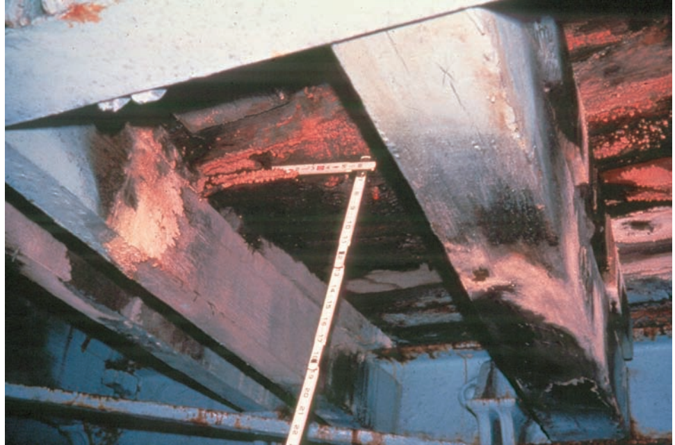
Figure 6.1.13 Decay in a Timber Beam
