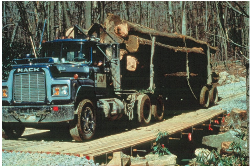
Figure 6.3.1 Stress-Laminated Timber Slab Bridge Carrying a 90,000-Pound Logging Truck (Source: Barry Dickson, West Virginia University)
