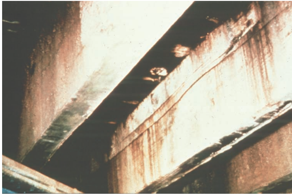
Figure 6.1.12 Horizontal Shear Crack in a Timber Beam
